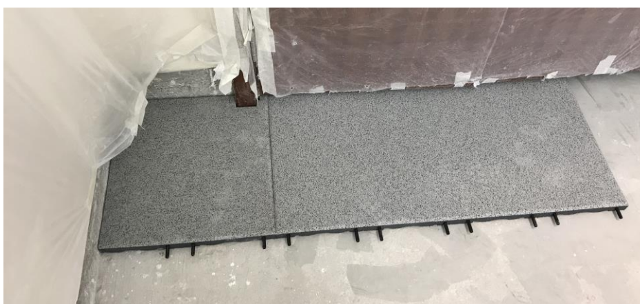
Installation of the tiles along a wall with the connector pins at the front
